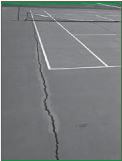
Cracked tennis courts Canchas de tenis quebradas
